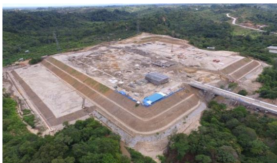
275/33 KV Substation at Lambir for SEB
